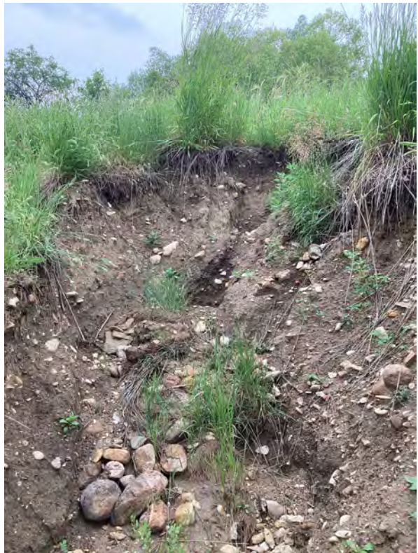
2.4 Holly No. 1 Reservoir - Erosion on North End of Dam On East Side (Looking Southwest)
