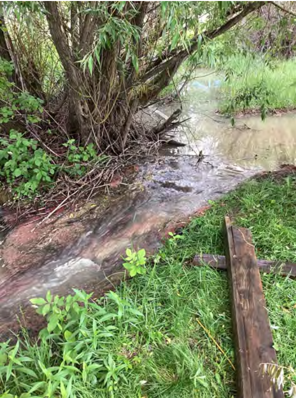
1.3 Sheridan County Fairgrounds Reservoir - Eroded Spillway (Looking Southeast)
