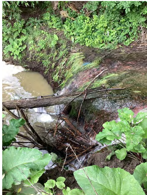
10.4 Unpermitted Reservoir - Emergency Spillway Erosion (Looking South)
