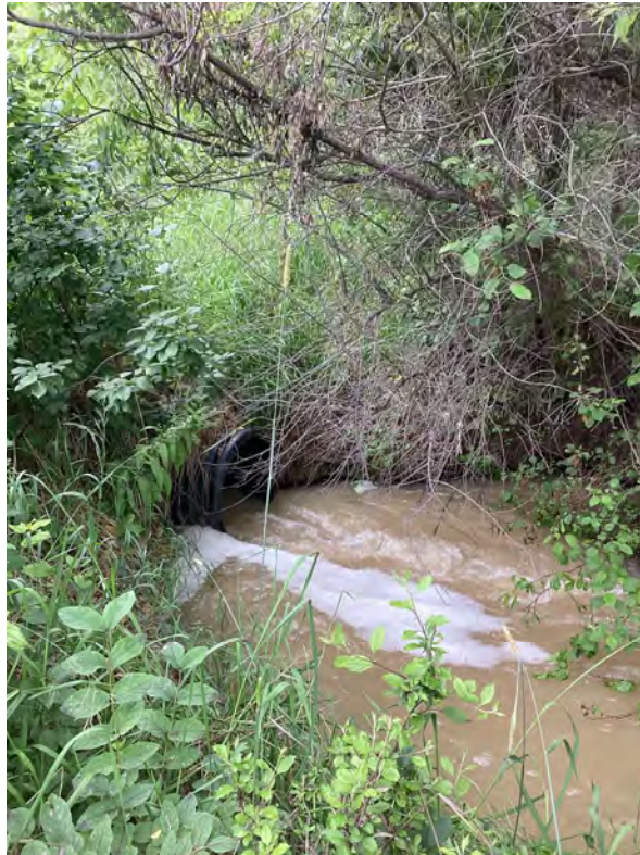
4.3 Holly Ponds No. 4 Reservoir - Outlet On Downstream Side of Dam (Looking North)
