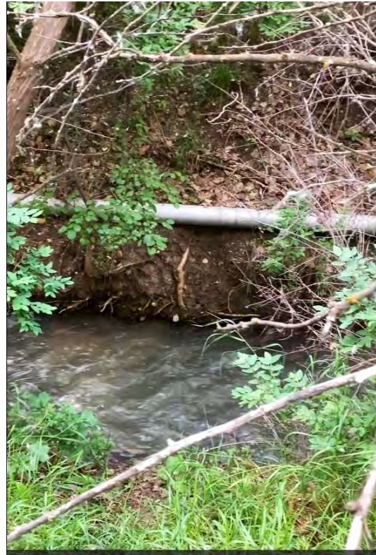
12.4 Hume No. 3 Reservoir - Dam Breach (Looking South)
