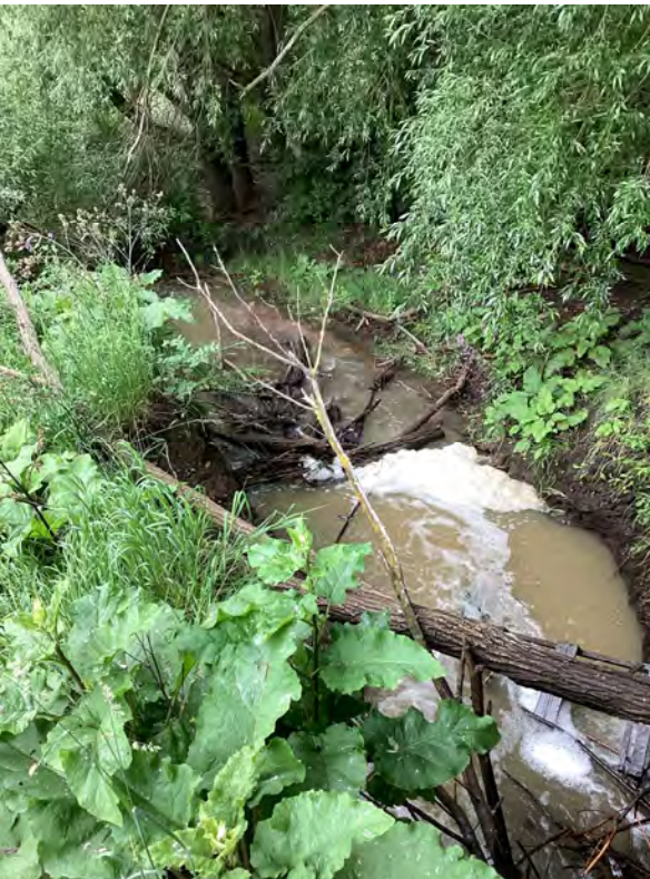
10.3 Unpermitted Reservoir - Emergency Spillway Erosion (Looking South)
