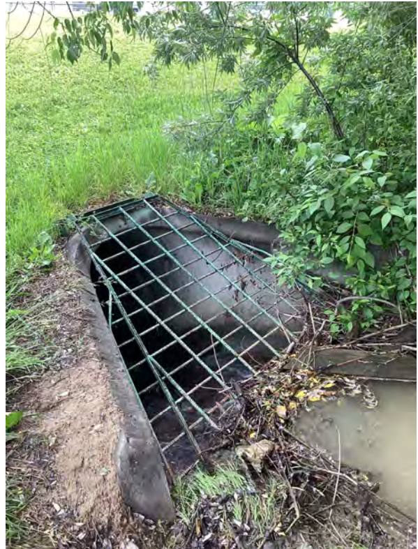
1.3 Sheridan County Fairgrounds Reservoir - Eroded Spillway (Looking Southeast)
